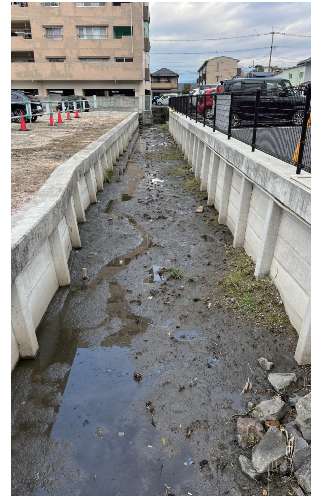
Figure 79 Monotone edge by concrete
