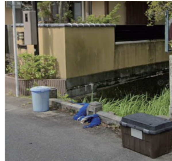
The canal flowing between the elementary school and the houses is overgrown with grass. The bridge is garbage dump now.
