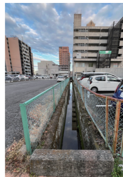
Figure 122 Parking lot and water in commercial area
