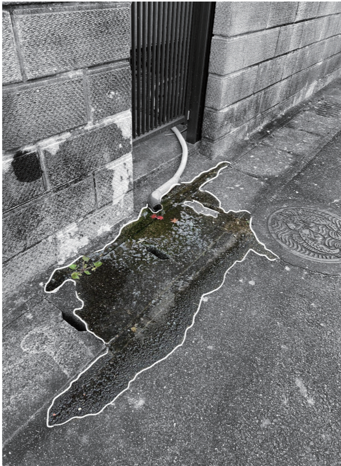
Figure 56 Waste water running to the ditch
