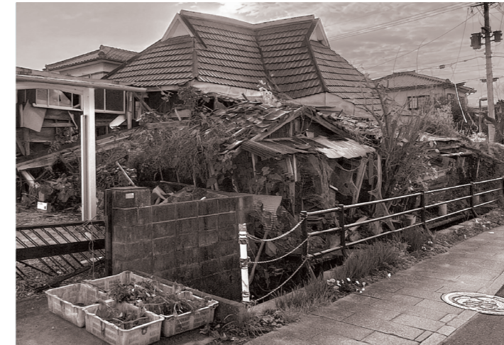
Figure 2 A vacant house in Saga, Japan
