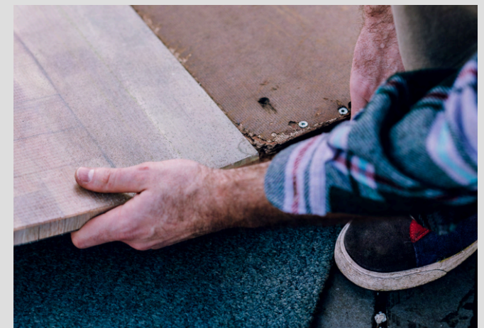
Figure 113: good tolerances in the track surface between joining edges
