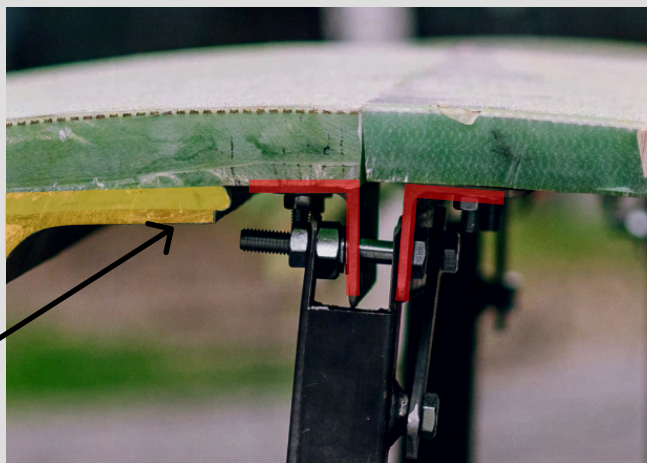
Figure 112: excessive shear web glue obstructing the positioning of the L-profile
