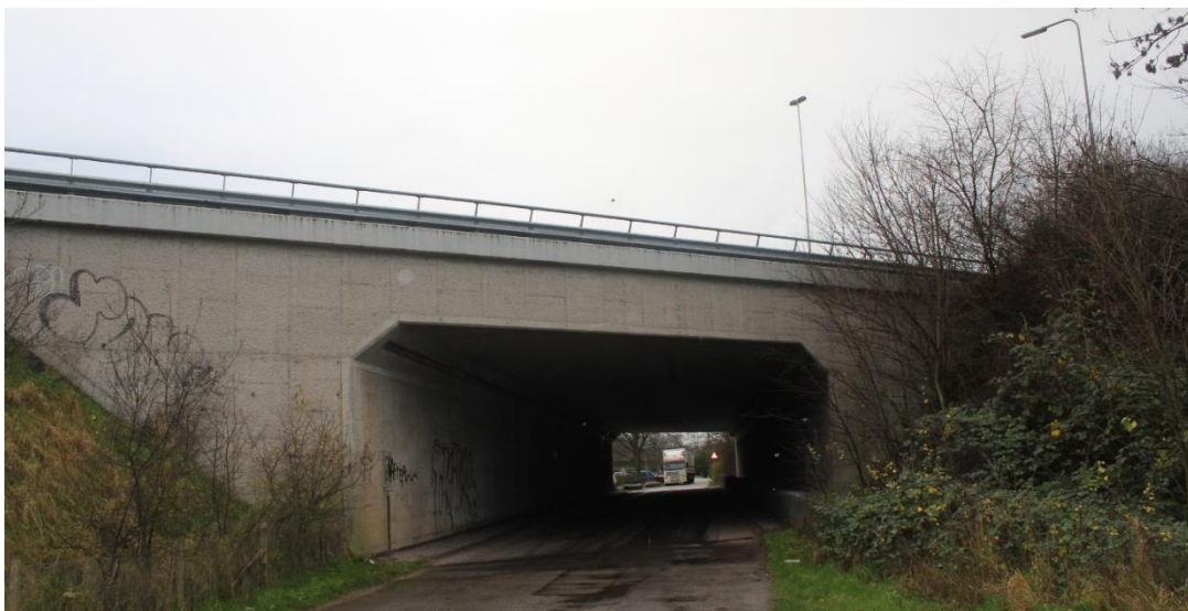
Figure 7 Example of a box-shaped reinforced concrete underpass situated in the A27 near Utrecht constructed in 1970 (from RHDHV)
