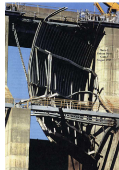
Figure 1.2: Close-up of the Tainter-gate after failure [9]
