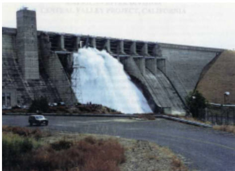
Figure 1.1: Folsom dam after the Tainter-gate failed [9]
