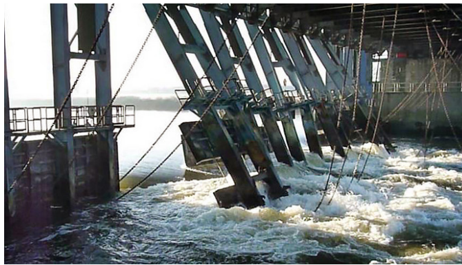
Figure 1.4: The broken weir at Grave
