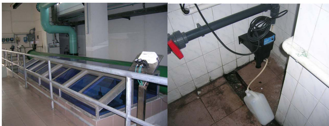
Figure 3-1 Filters and Water Sample at Intake, Taihe Water plant
