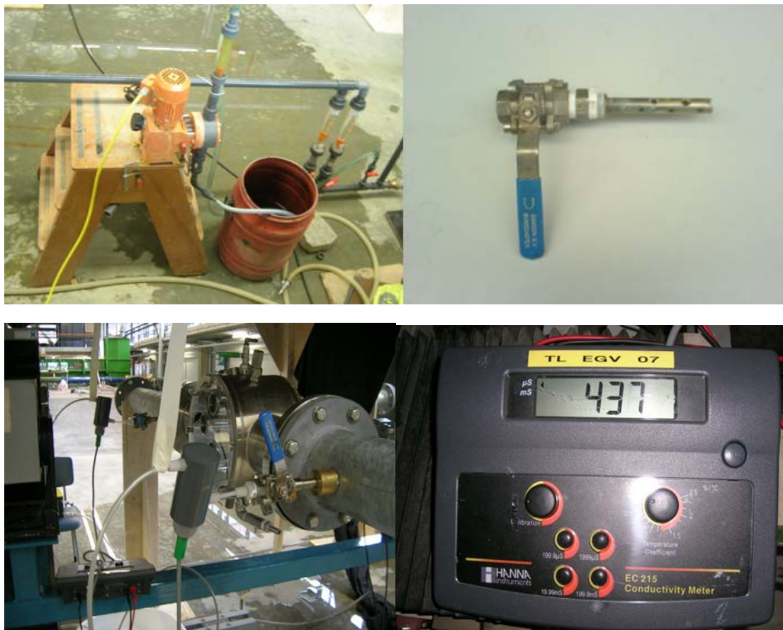
Figure 6-13 Dosing vessel and dosing pump (top left); Insert pipe (top right); Salt dosing set-up (bottom left); conductivity meter reading (bottom right)
