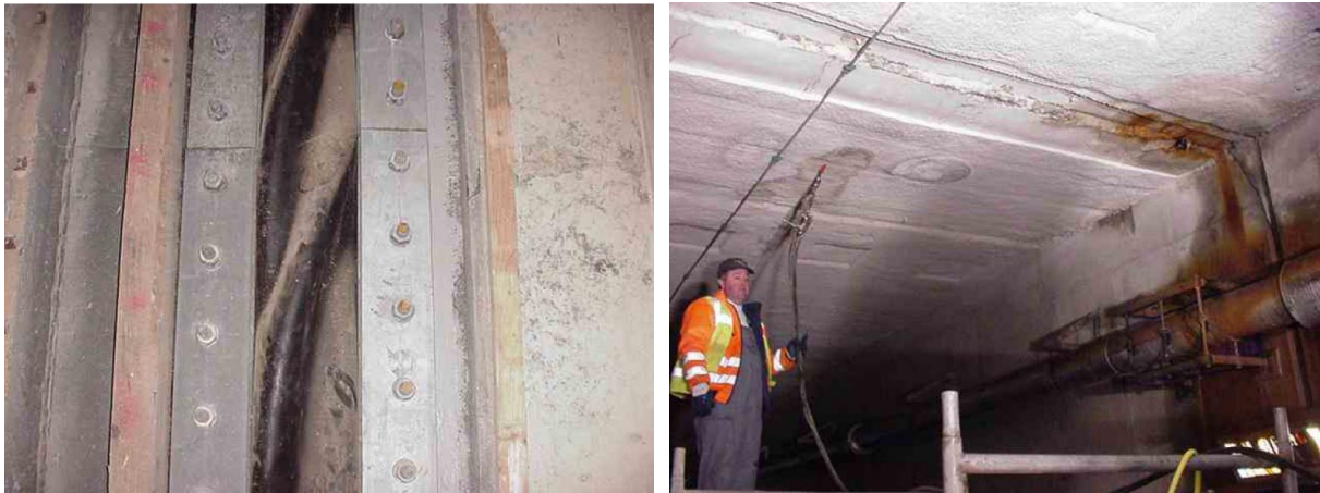
Figure 2.32: The deformed OMEGA-profile (left) and the leakage and repair in the metro tube (right). [39]
