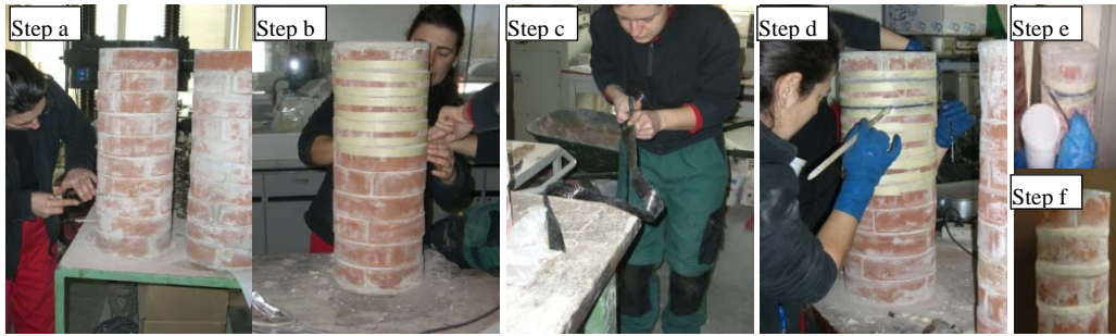
Figure 4: steps for the strengthening with repointing technique (step a: cleaning, step b: protection of brick elements, step c: cutting of carbon fibers, step d: application of epoxy resin and layers of fibers, step e: application of quartz grains, step f: application of mortar).
