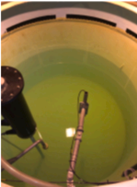
Fig. 11. Full-scale pellet softening reactor top view, reactor diameter ( D = 2.6 m).
