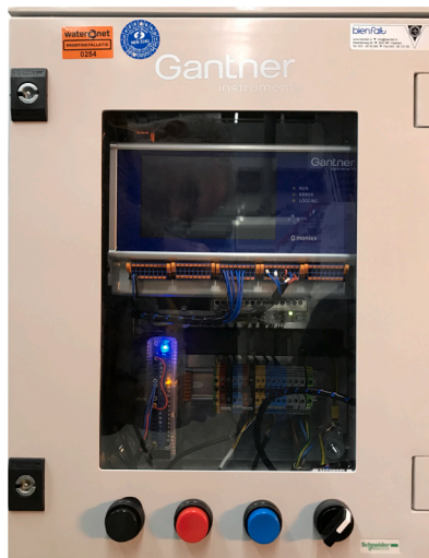
Fig. 5. Data transfer unit.
