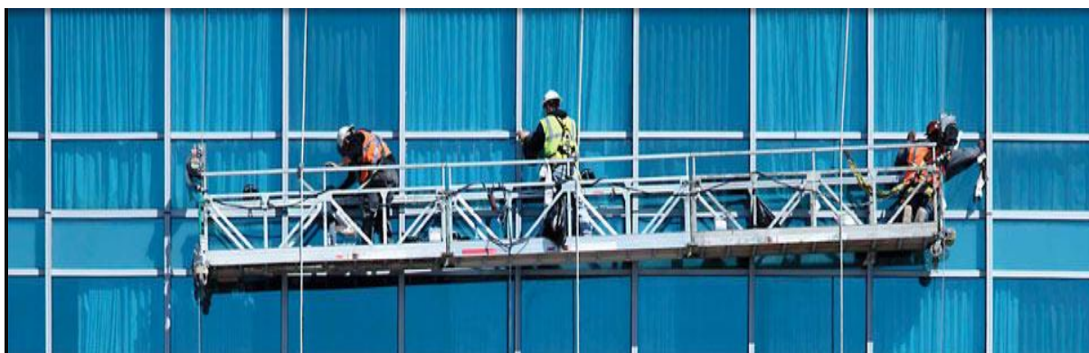
Figure 18 Suspended access platform, an example of exterior working station to support selective demolition work. (Source: Jeevan suspended platform)
