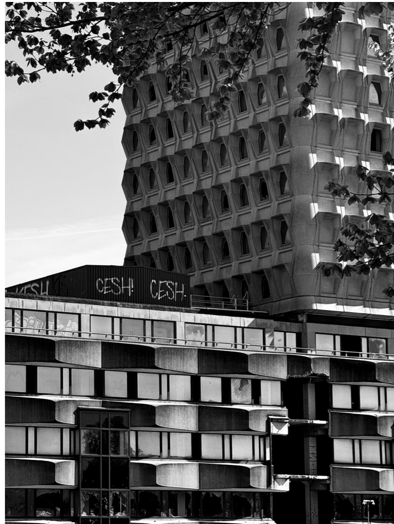
FIGURE 41: NORTH-WEST SIDE OF THE DAMAGED FACADE
