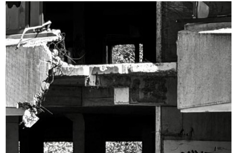
FIGURE 59: EXPOSED AND DAMAGED PREFAB ELEMENT AND FLOOR SLABS AT THE DAMAGED LOCATION
