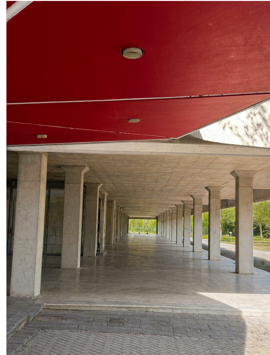
FIGURE 51: IMPRESSION OF THE GROUND FLOOR IF CLEANED (GRAFFITI REMOVED)
