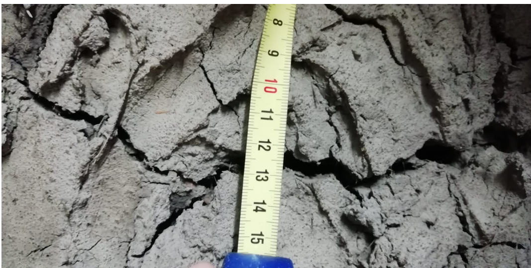
Figure B.7: The clay sample after 110 hours, detailed image of the largest fracture with tape measurer in cm for scale.
