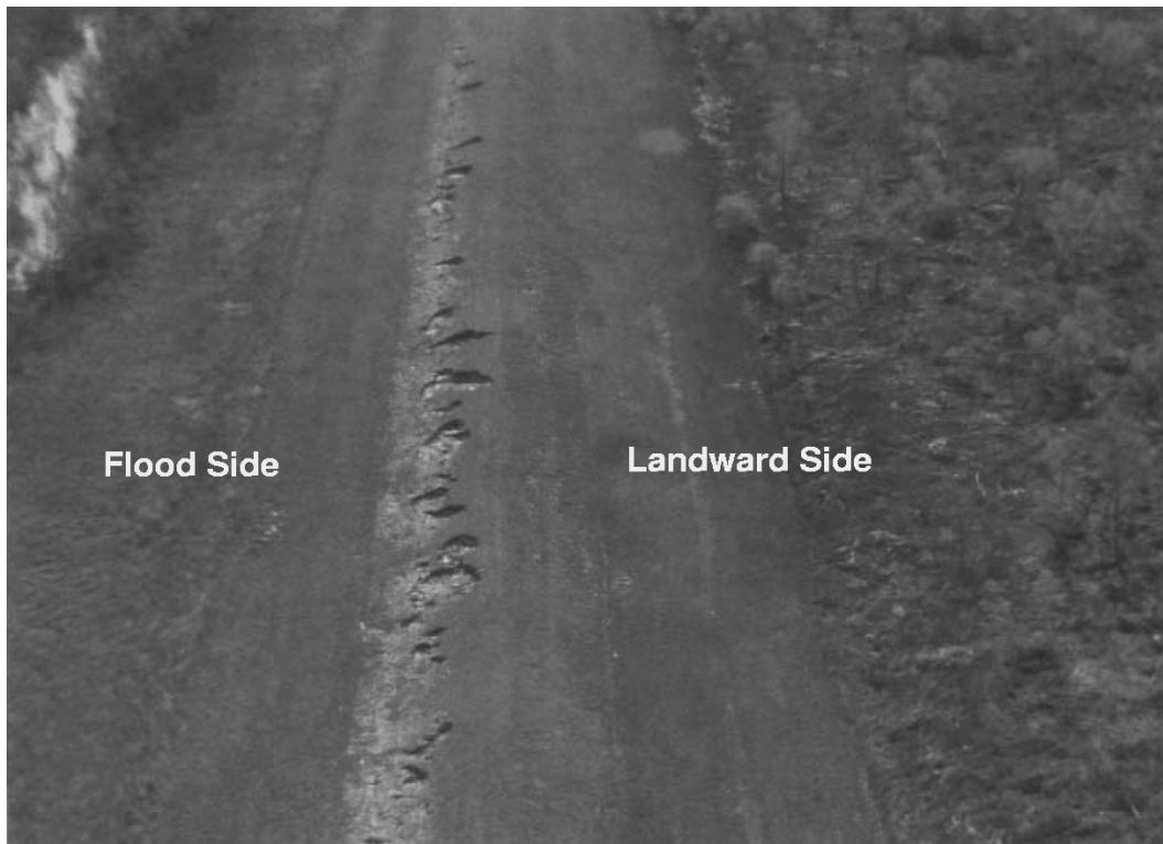
Figure 1. Wave damage on flood side of MRGO levee facing Lake Borgne.
