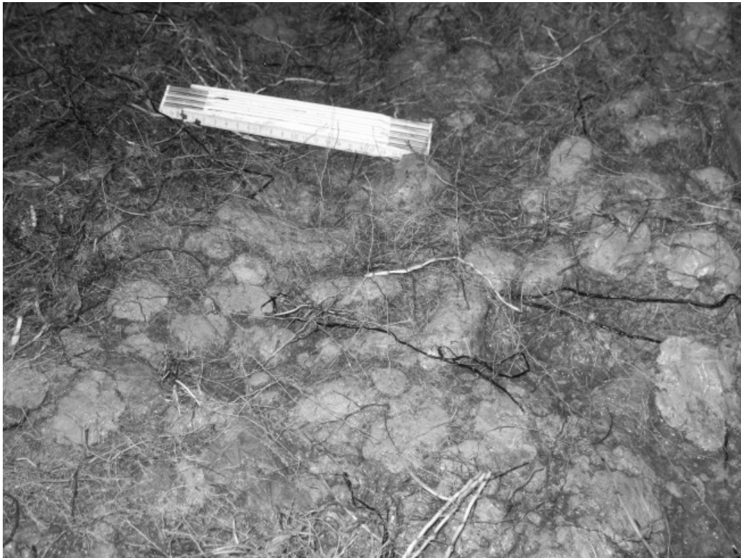
Figure 13. Damage to the cover layer in the breaker zone (from Geisenhainer 2008).
