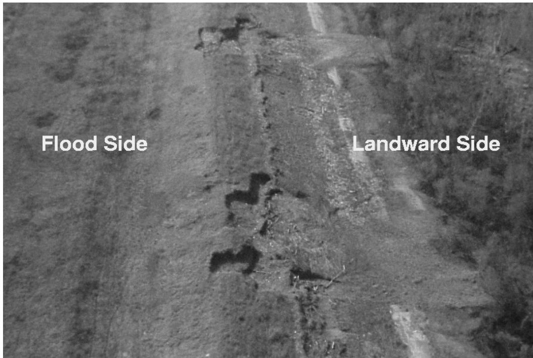
Figure 2. Wave overtopping or surge overflow damage on landward side of MRGO levee.
