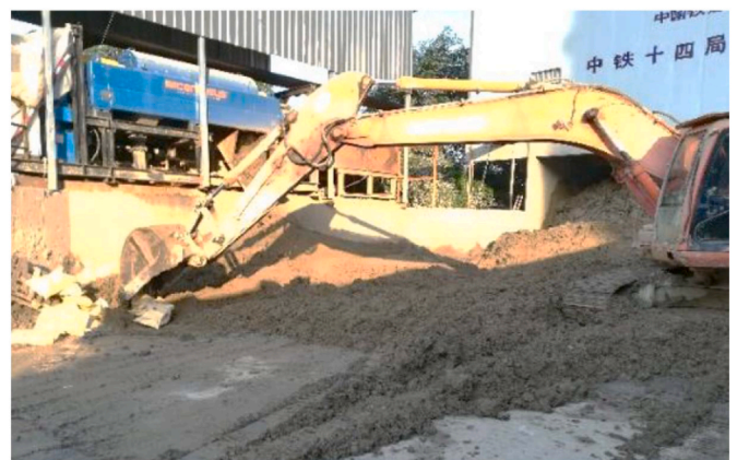
Fig. 15. Stockpiling of discharged soil from shield tunnel construction (Zhang et al., 2022a).
