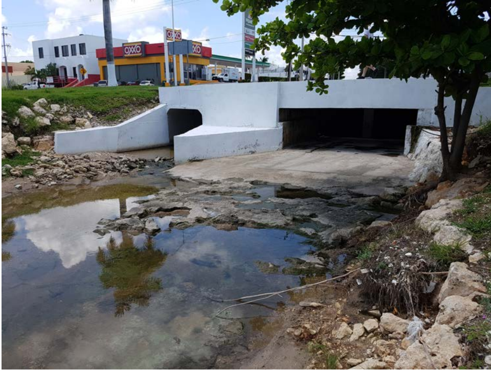
Figure G.5: Outlet of drainage system near the university
