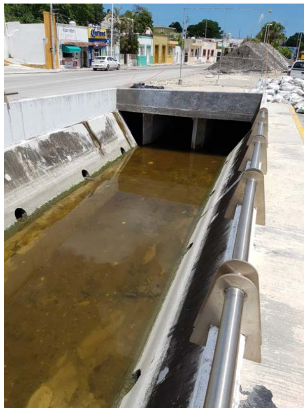
Figure G.2: Ría of the drainage system near Calle 10
