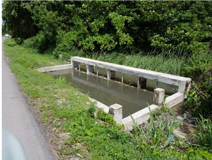
Figure G.1: Outlet of drainage system in Los Petenes
