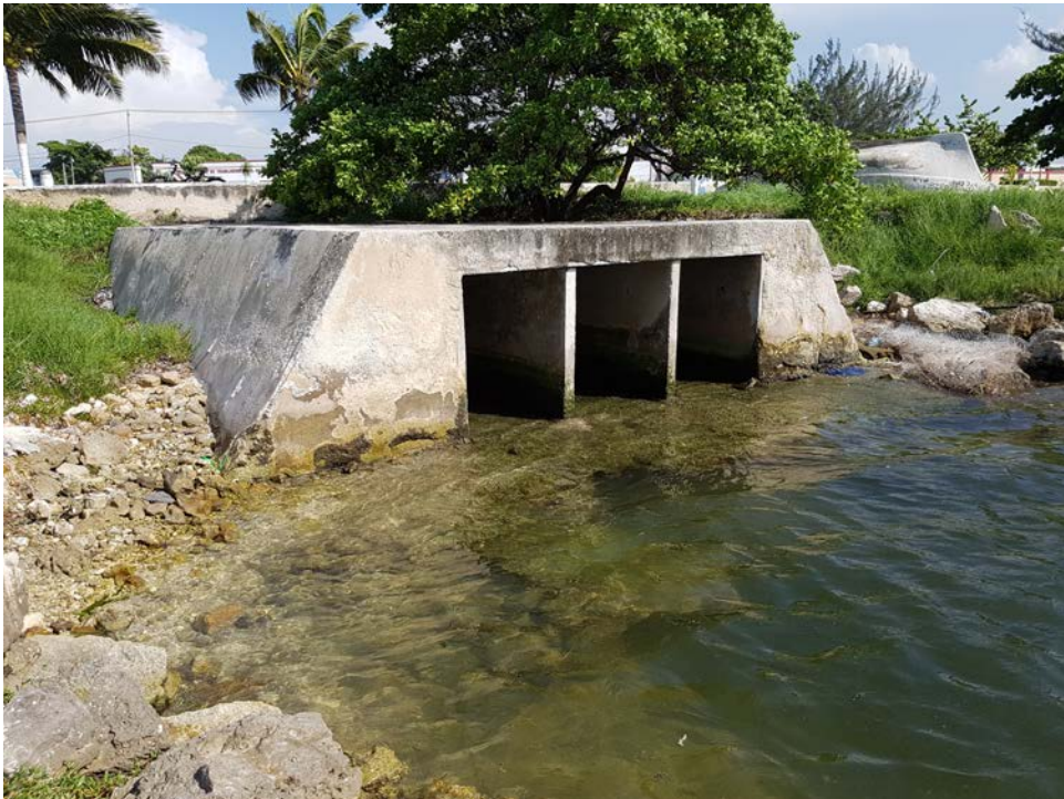
Figure G.4: Outlet of drainage system near San Roman barrio
