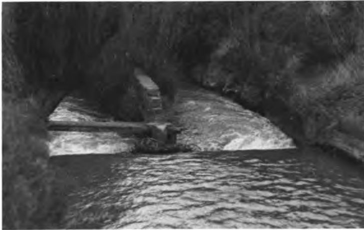
Photo 2. Sharp-nosed intermediate piers tend to trap floating trash.
