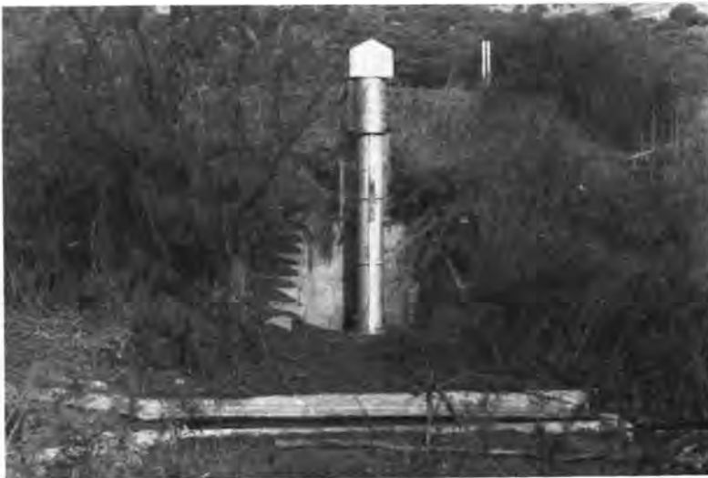
Photo 3. A stilling well made of steel pipes.
