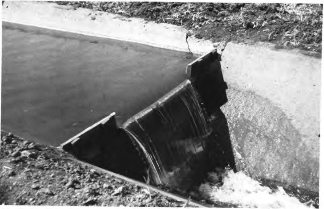
Photo 1. Rectangular sharp-crested weir.
