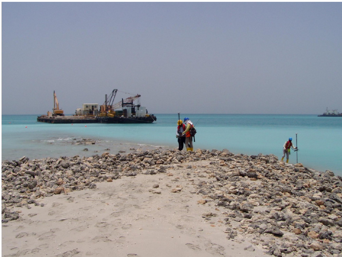
Figure 1.1 – Survey on a reclamation bund partly washed away by a storm in Khalifa (UAE) (picture by Royal Boskalis Westminster nv)
