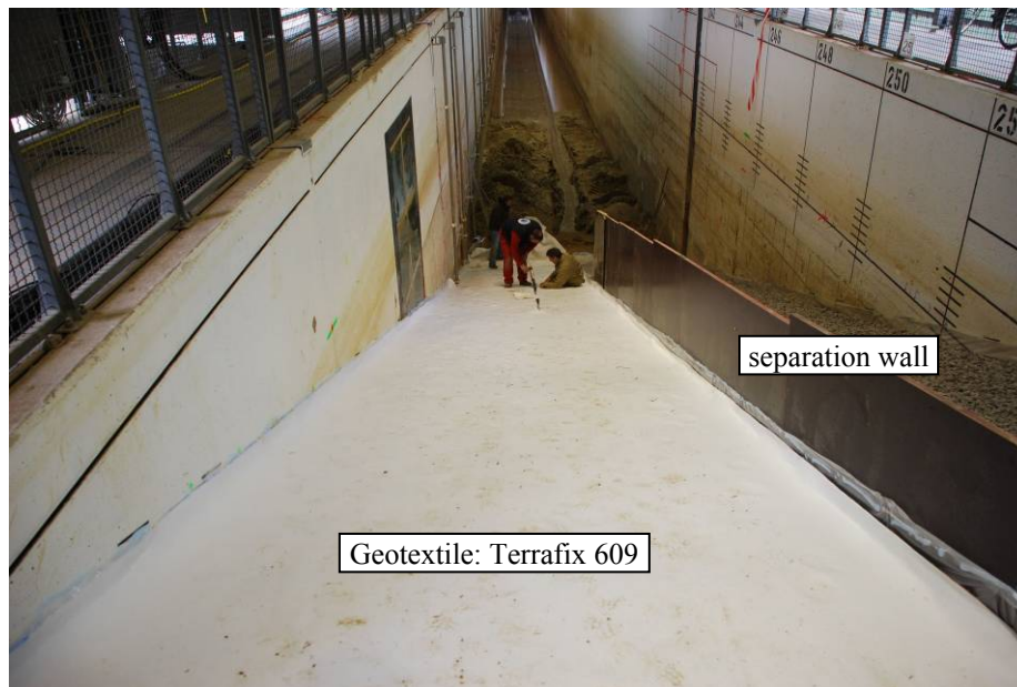
Fig. 2.9: Geotextile placed beneath the revetment and extended at the side walls and the separation wall
