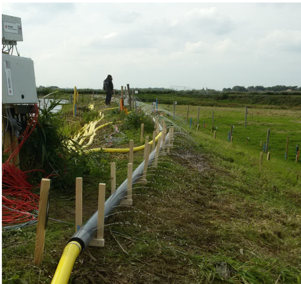
Figure 2.11: Dyke wetting system.
