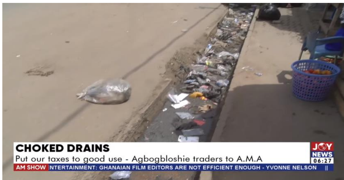
Figure 14: Choked drains at Agbogbloshie market (AM News on Joy News (20-5-22))
