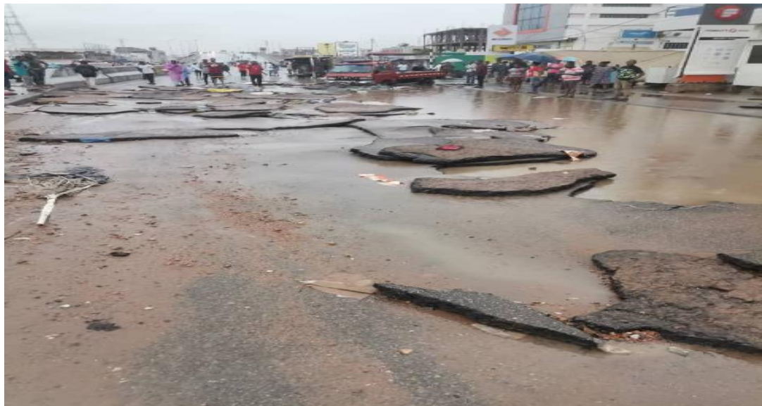
Figure 2: Aftermath of May 24 Flooding at Abossey Okai source (Daily Graphic (2022))
