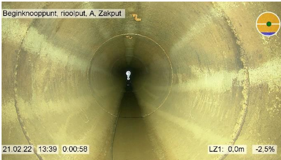
Figure 13: An impression of the sewer pipe at test set-up B, view from starting node
