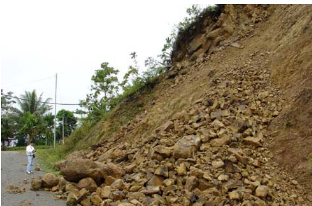
Figure 1 Rock slope failure on road cut slope due to stress changes and weathering.
