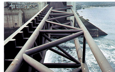
b) Support structures of hydraulic barriers
