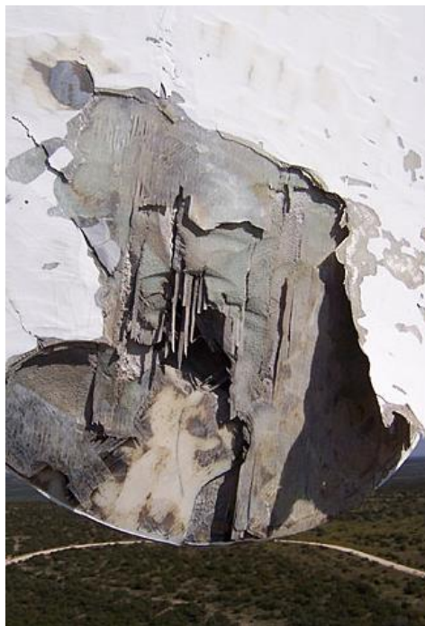
Picture 31. Damage due to a lighting strike. Picture from betterplan.squarespace.com, (2009).
