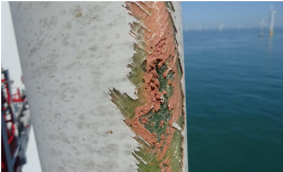
Picture 29. Leading edge erosion on an offshore wind turbine blade (stateofgreen.com, 2023).
