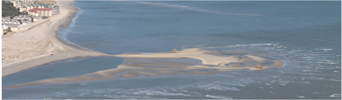
Figure 10.3: Picture taken from the air. On this picture, two excavators are visible, scraping the incoming shoal and loading the sand into dump-trucks which take the sand to the erosion hot-spots on the other sides of the beach. To get on the shoal, a small bridge was build and work was only possible during low tide.
