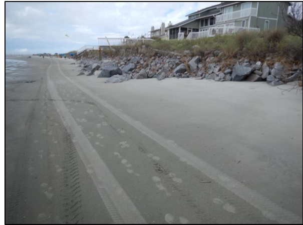
Figure 10.8: Exposed revetments along the IOP coast between 42nd and 53rd Avenue (source: CSE)
