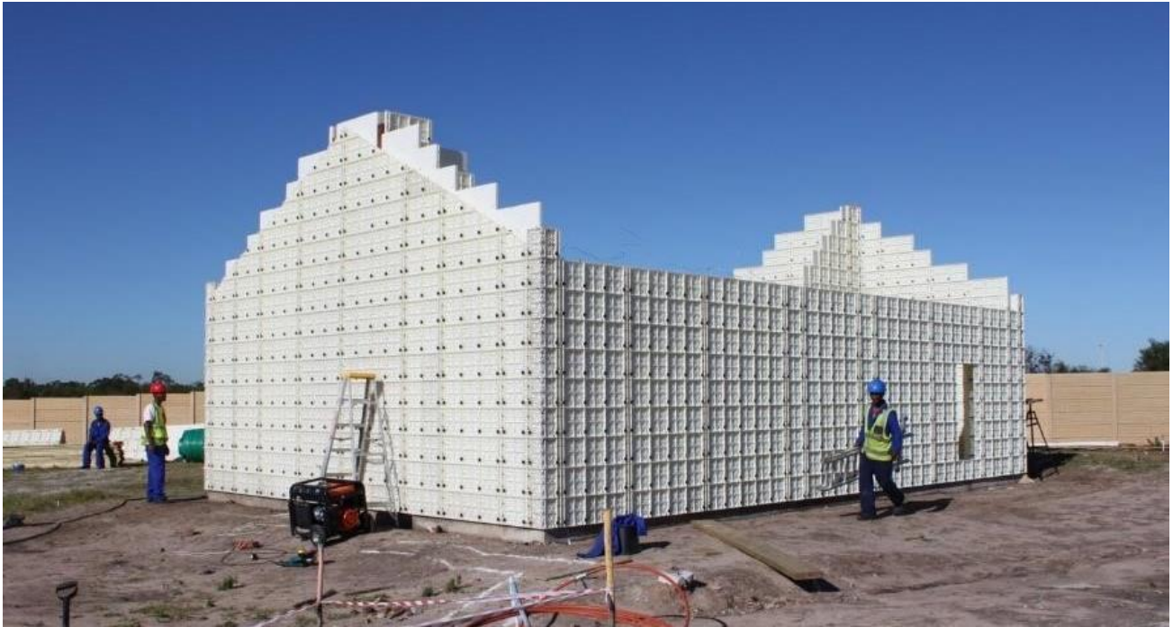
Figure 56: Moladi mould system on a building site (Engineering For Change | By Engineers, For Everyone, 2020).
