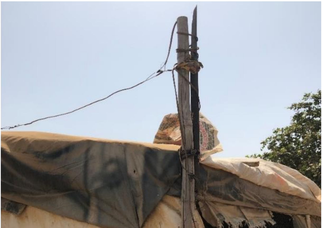
Figure 27: Electricity supply wires connected by bamboo poles.
