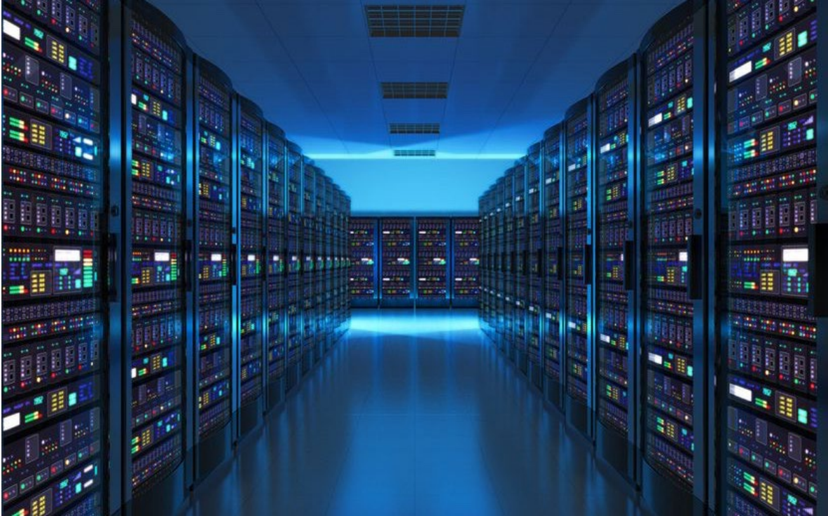
Figure 3 The interior of a Cloud data centre or so-called ‘server farm’ (Laboratorio Linux, 2017, https://creativecommons.org/licenses/by-nc-sa/2.0/ ).
