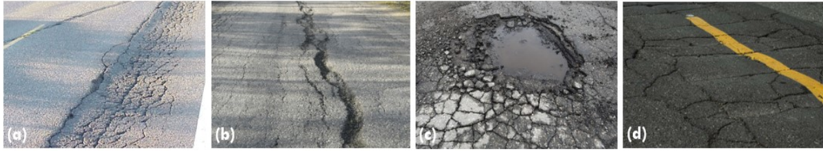
Figure 2.16: Other types of distresses in asphalt. (a) Rutting; (b) upheaval; (c) potholes; (d) corrugation and shoving
