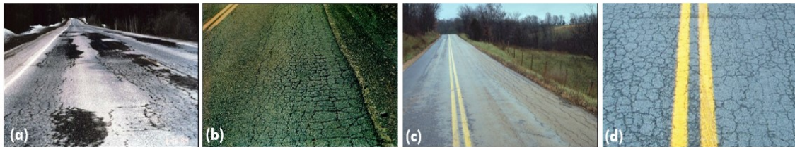
Figure 2.17: Various fatigue cracks [53] due to (a) frost; (b) load cycles; (c) lack of edge support; (d) cyclic loads
