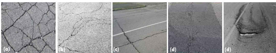
Figure 2.15: Different crack patterns. (a) Fatigue cracks; (b) block cracks; (c) transverse cracks; (d) reflective cracks; (e) slippage cracks
