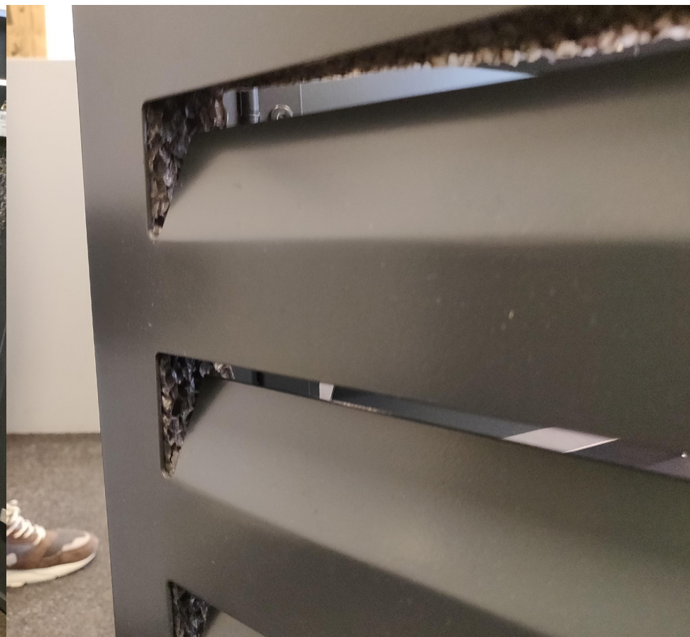
Figure 34: Foam being visible through the side of the lamellas
