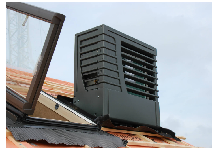
Figure 7: Example of a roof mounted heat pump (Ubbink, n.d.)
