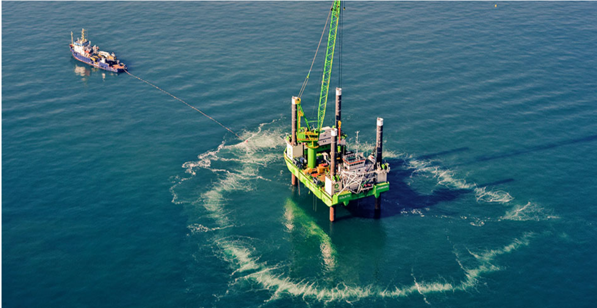
Figure 2.4: Hydrotechnik Lübeck: the Big Bubble Curtain with a jack-up vessel by at the OWF Borkum West II (Photo: Trianel / Hero Lang)
