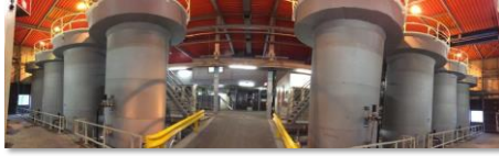
Full-scale drinking water pellet-softening reactors
