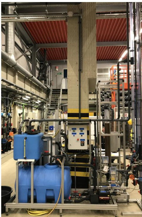
Figure 9 Waternet expansion column in Amsterdam
