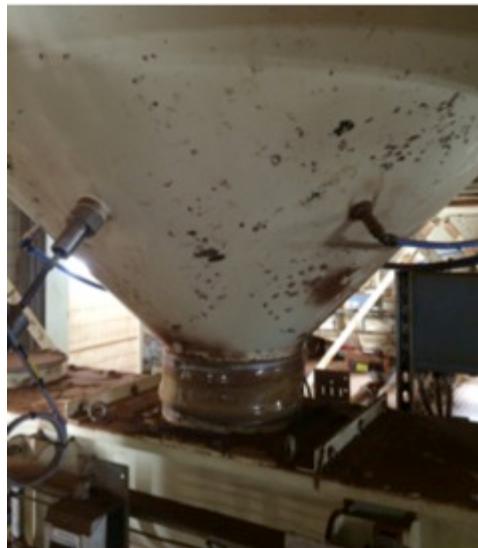
Fig. 3.12. Hammer marks on the converging part of the silo
