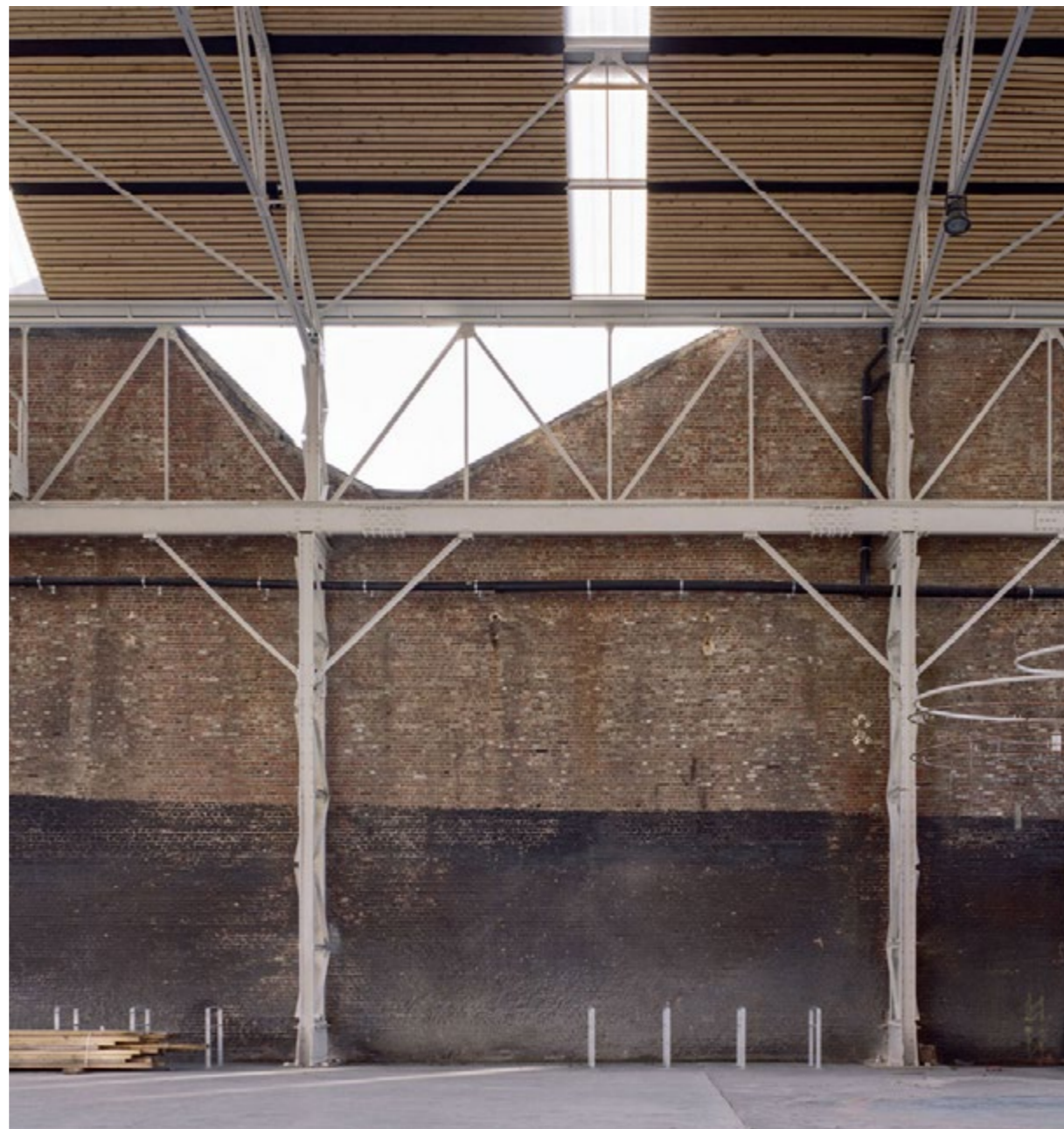
Atelier building in its current condition. No windows, no doors, just a blank facade.
