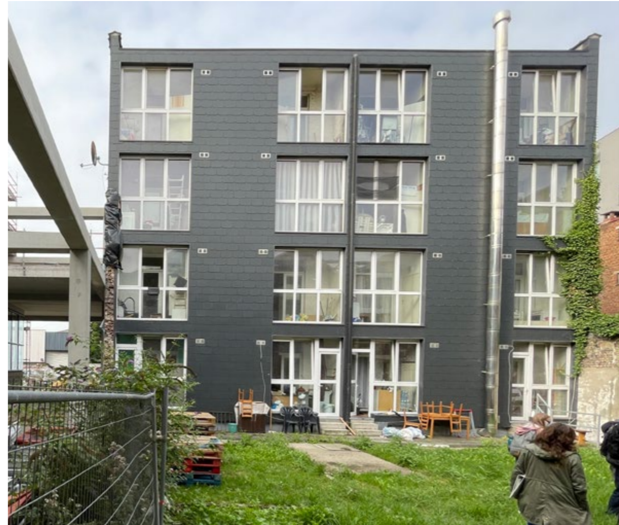
Photograph of the current state of building B's facade that is facing the social court. The facade here is completely different compared to the previous ones. A cheap modification that happened over time, but something that gives more flexibility to work with. The big windows are intriguing and receive lots of light in the afternoon hours. This facade used to have balconies where the big windows are located but they were converted into indoor spaces by the residents.
