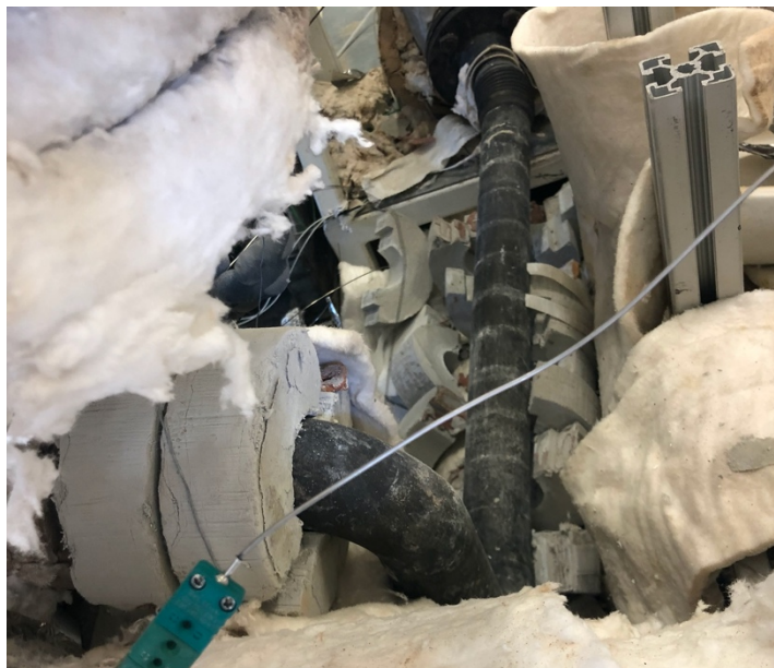
Figure 31 Defect pipe section between tar reformer and afterburner stripped down and checked for leaks. This was causing the tar reformer to not be able to reach its operating temperature and eventually delayed the test runs.
