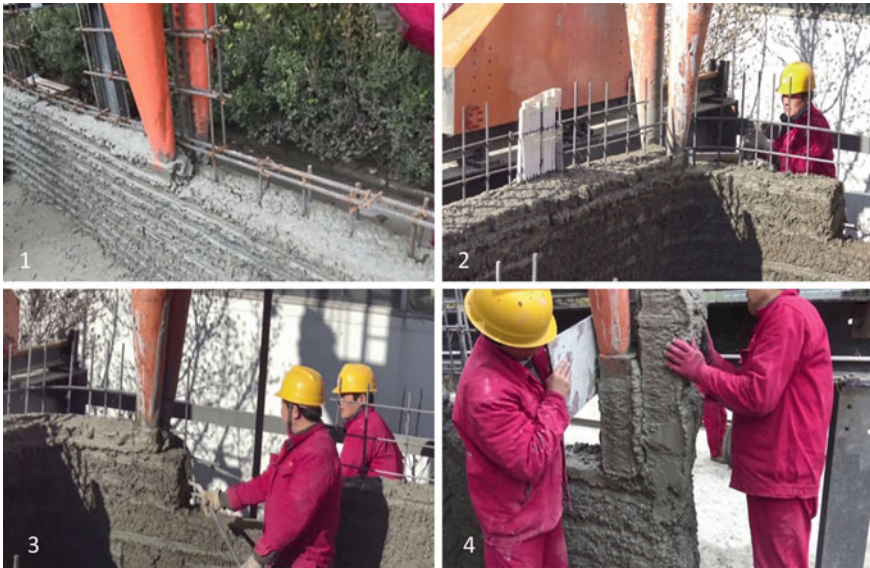
Fig. 2.24 Construction of the two-storey villa: 1. forked nozzle lays concrete on both sides of the rebars, 2. printing a bow; 3. manual help at the opening, when the material flow is interrupted; 4. forming a vertical element
