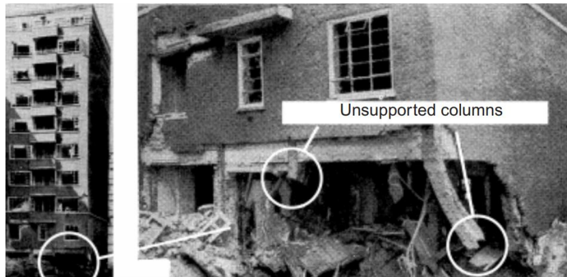
Figure 2.5: Compressive strut action carries additional gravity load after two columns failed during WW2 [28].
