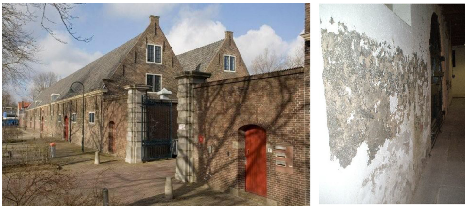
Fig. 1. Paardenmarkt (Delft, Netherlands), exterior and damage in the interior.
