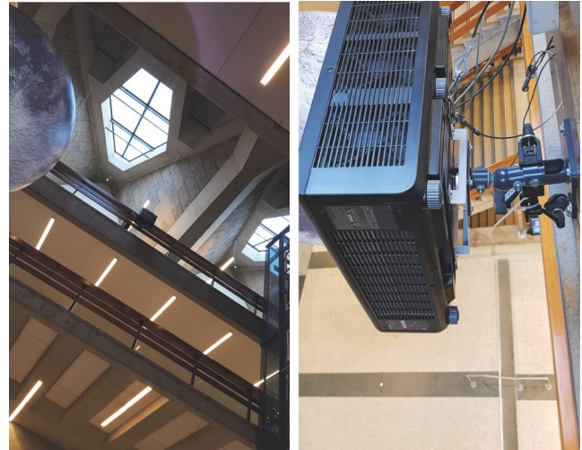
FIGURE 3: IMOVE setup and installation location.
