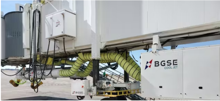
Figure 2.4: Jet bridge with PCA and GPU units 3
