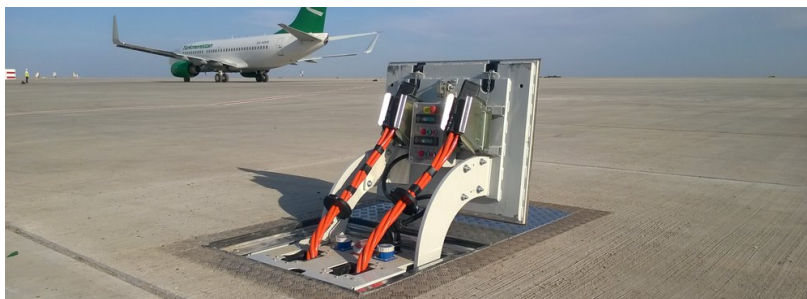
Figure 2.6: Ground power pit 4
