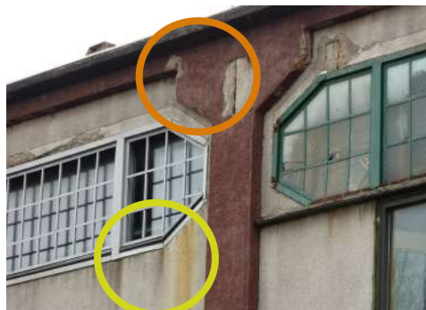
Damage on concrete - rebars`
