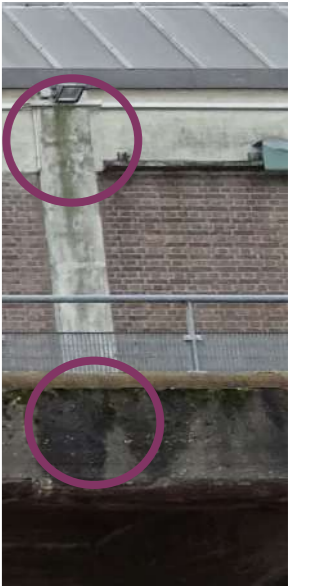
Moist spots and biologic growth
