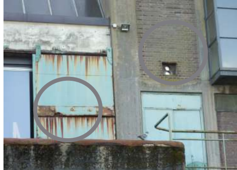
Damage on steel and brick
