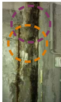
Moist spot - Damage on rebars
