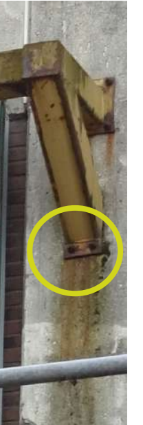
Rust staining on concrete
