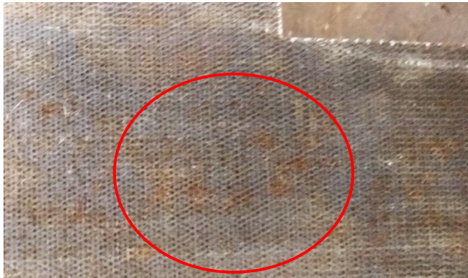
Figure A.0.5: Non-localised Corrosion of Steel due to Water Ingress from Cutting Attempt
