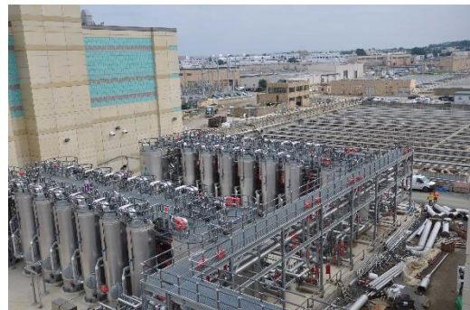
Figure. 9 Bio-gas installations Photo
