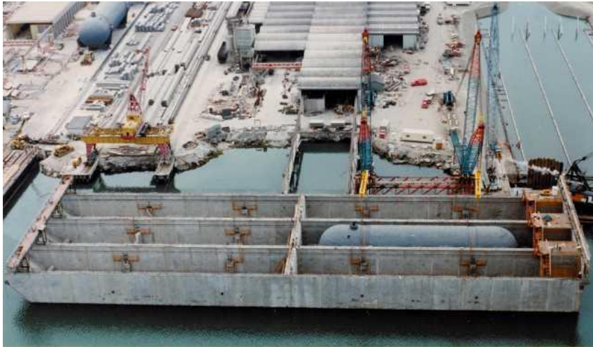
Figure 6.8: Construction of a concrete LPG floating storage facility, Java sea, Indonesia [W24]
