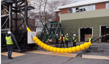
(a) Cable protection system [W11]
