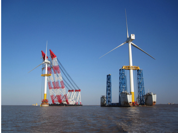
(a) Full pre-assembled turbine [W6]
