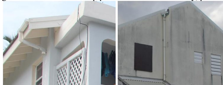
(Rainwater collected by gutter enters an open pipe, photo by author)
