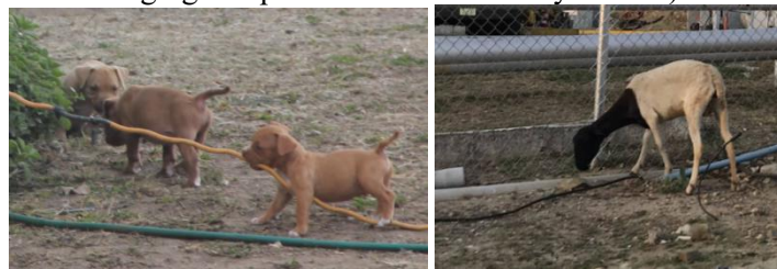
(The exposed water pipes are easily damaged by animals. Photo by author)
