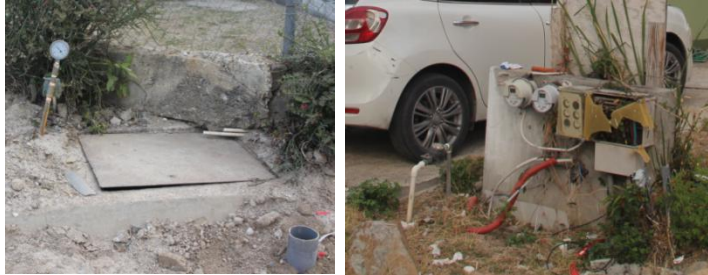
(Left: The water supply pipe exposed to the external environment is extremely vulnerable; Right: Aging and poor facilities. Photo by author.)
