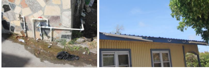
(Left: Water supply pipe that is leaking; Right: Gutter which was damaged by the hurricane. Photo by author)
