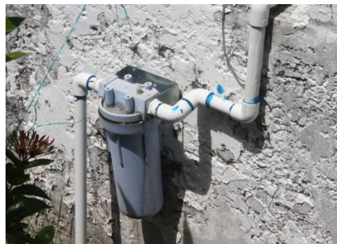
(The filter which connect the pipe and GEBE water pipe, photo by author)
