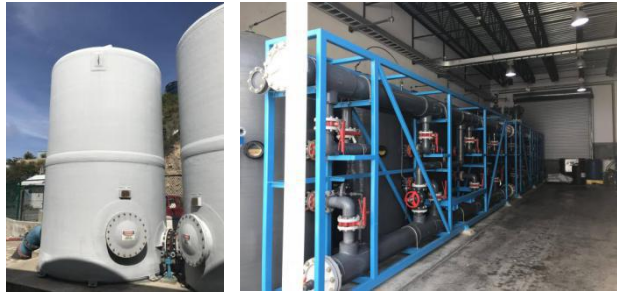
(Freshwater storage tank and energy recovery system, photo by author)
