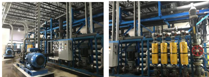
(The reverse osmosis membrane stack system, photo by author)
