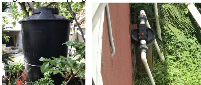
(The tank and filter. Photo by author)
