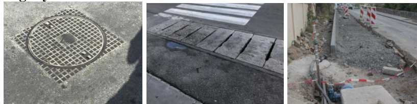
(Urban sewer ditch, well and drainage pipe. Photo by author)
