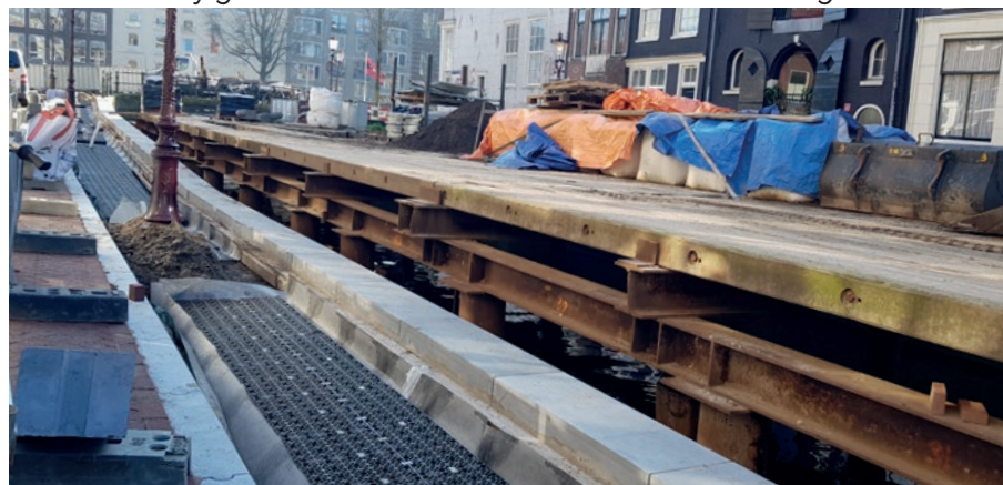
Image 4.5 Before (left) and after (right) image of replaced quay wall waterfront at Rechts Boomssloot. Image credit: Noelle Teh
