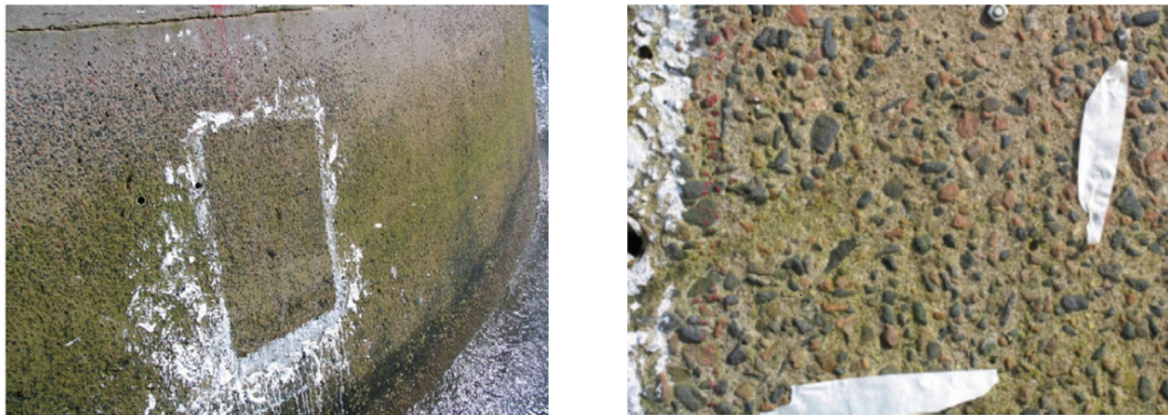
Figure 2.2: Abrasion by ice at concrete in Confederation Bridge at 0.3mm/year. [19]
