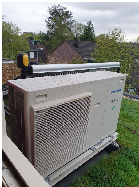
Figure 6.2: View from roof of retrofitted house. From left to right: solar boiler, heat pump and sedum roof cover (picture by first author).
