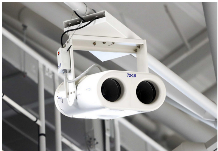
Blowers in the Olympic Oval of Gangneung (Spekenbrink, 2016)
