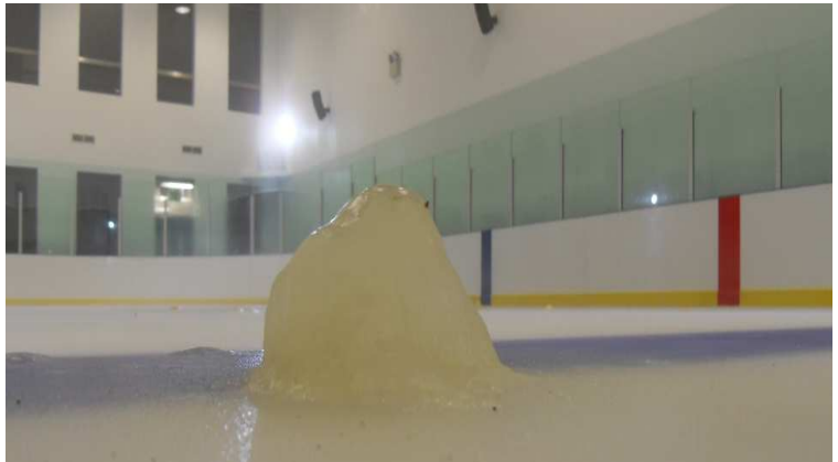
Condensated moisture drips from the ceiling onto the ice, which forms an ice stalagmite (Icerinksupply.com, 2017)
