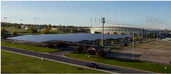
Solar panels installed above parking lot at the Utah Olympic Oval in Salt Lake City (Utah Olympic Legacy, 2017)
