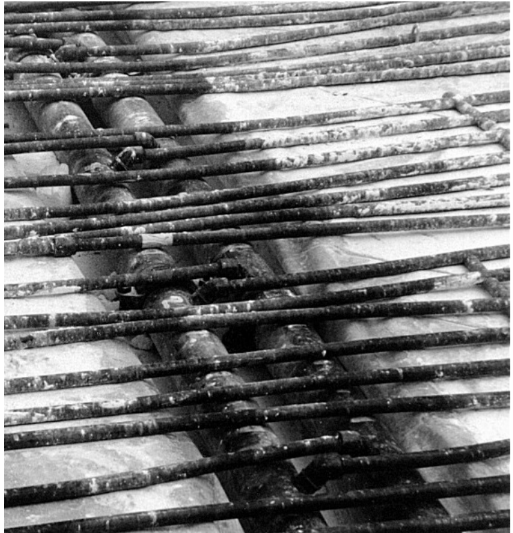
Im. 6.21: Refrigeration pipe system, which will be integrated in a concrete slab.
