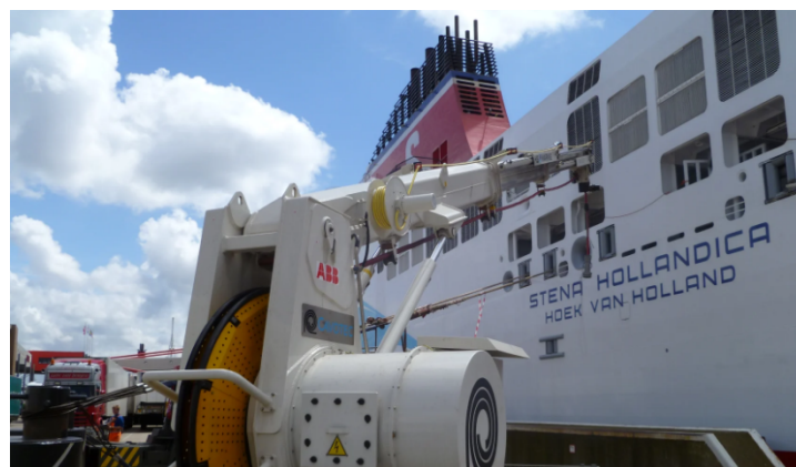
Figure 4.1: Visualisation of the cable connection between shore and ship at the Stena Line ferry terminal in the Port of Rotterdam (AMP, 2012)
