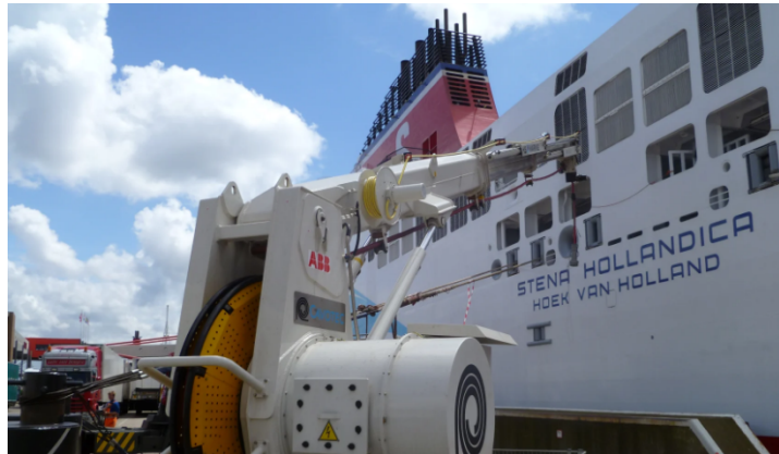
Figure B.2: The cable connection between shore and ship at the Stena Line ferry terminal in the Port of Rotterdam (AMP, 2012)
