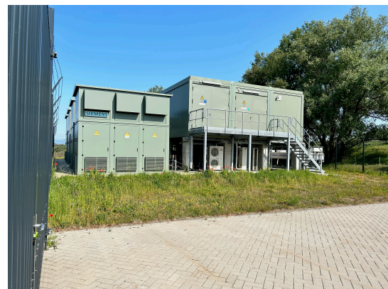
Figure B.7: Side view of the shore power installation of Heerema's offshore vessels Thialf and Sleipnir in Landtong Rozenburg
