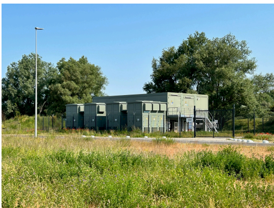
Figure B.6: Front view of the shore power installation of Heerema's offshore vessels Thialf and Sleipnir in Landtong Rozenburg
