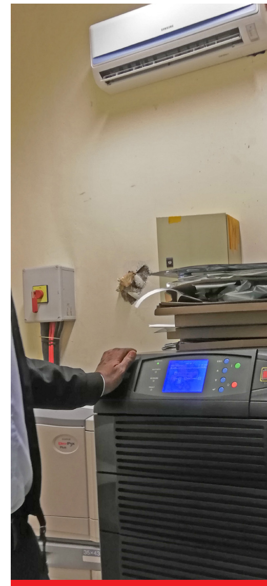
Figure 15. A back-up power supply unit for the CT-scanner in an air-conditioned room. Mbarara Hospital.
