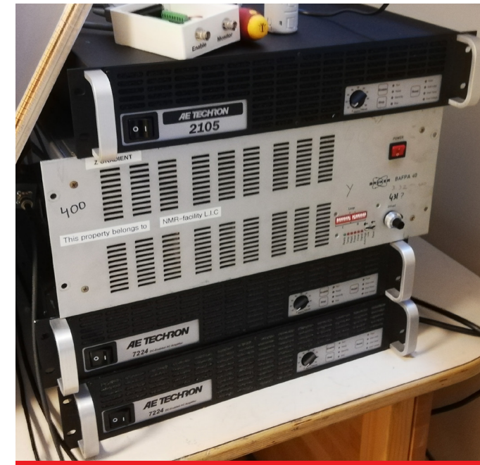
Figure 5. The current electronics setup. Black cases: gradient amplifiers. Silver case: RF amplifier.
