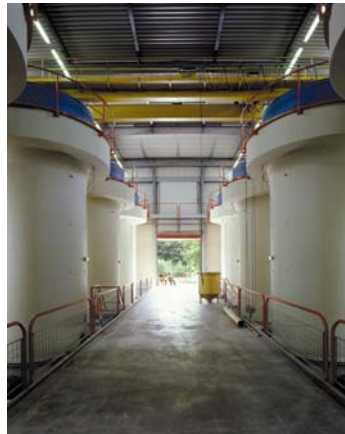
Figure 6.1 Pellet softening reactor
