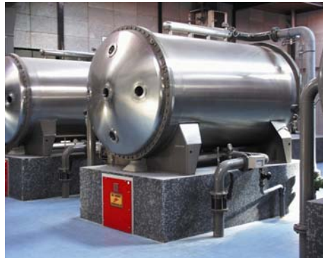
Figure 4.1 Ozone generator at Amsterdam Water Supply
